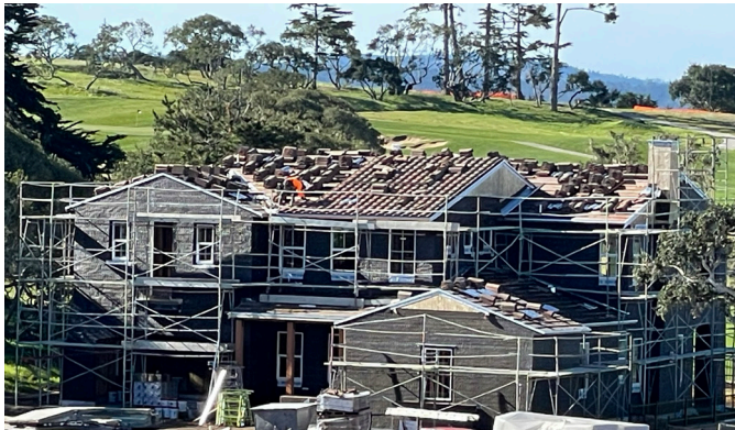
Fall protection is provided from the ground up on at the Enclave project.
